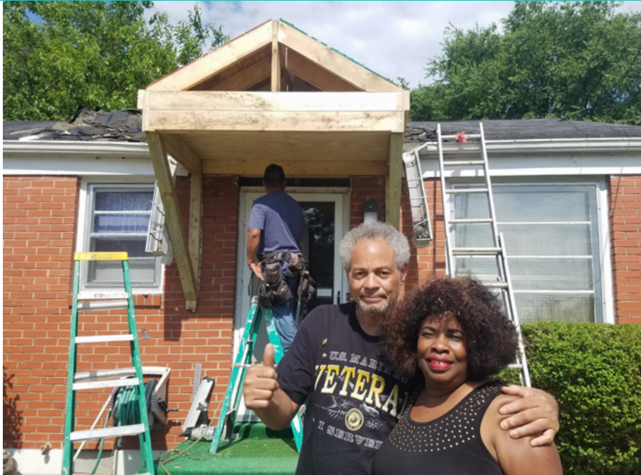
With funding from The Barnes Fund, Rebuilding Together repaired the roof and front entry on the home of Ms. Smith and her husband in 2019.
